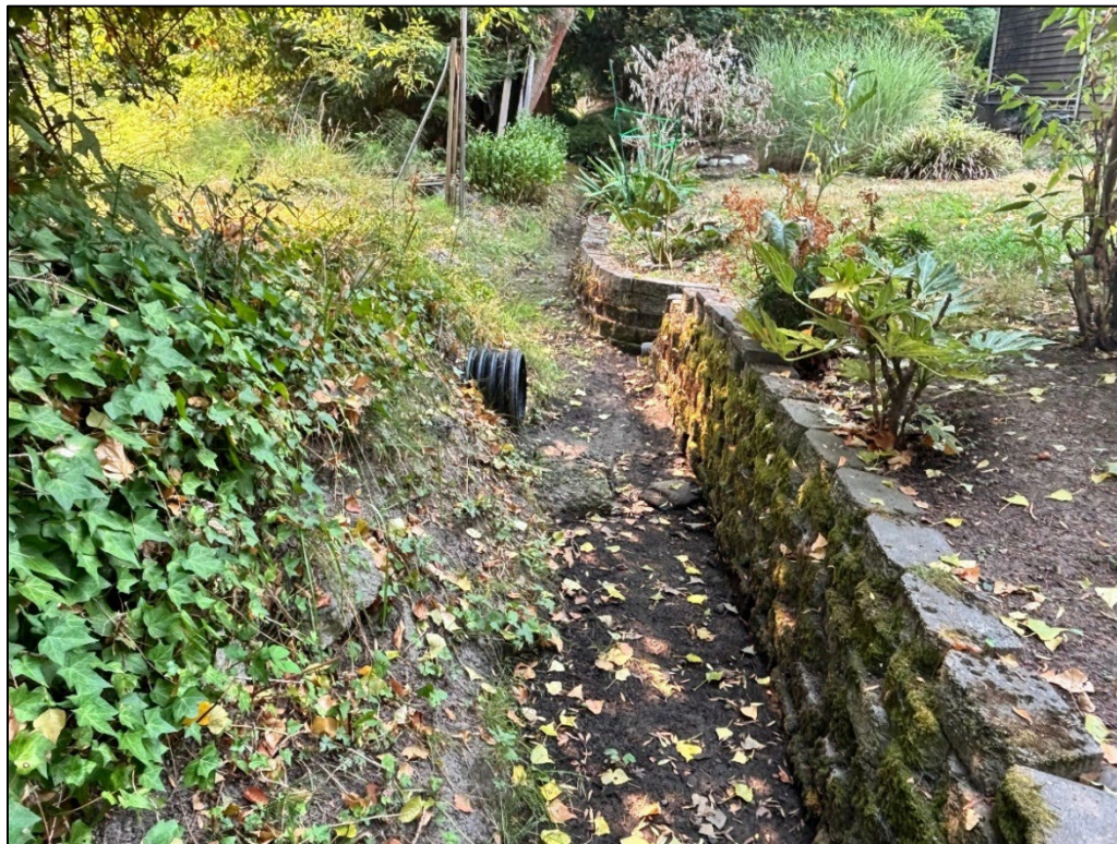
Figure 2. Location of the mapped transition point from stormwater ditch to open watercourse, viewed from southeast corner of subject property, facing south.
