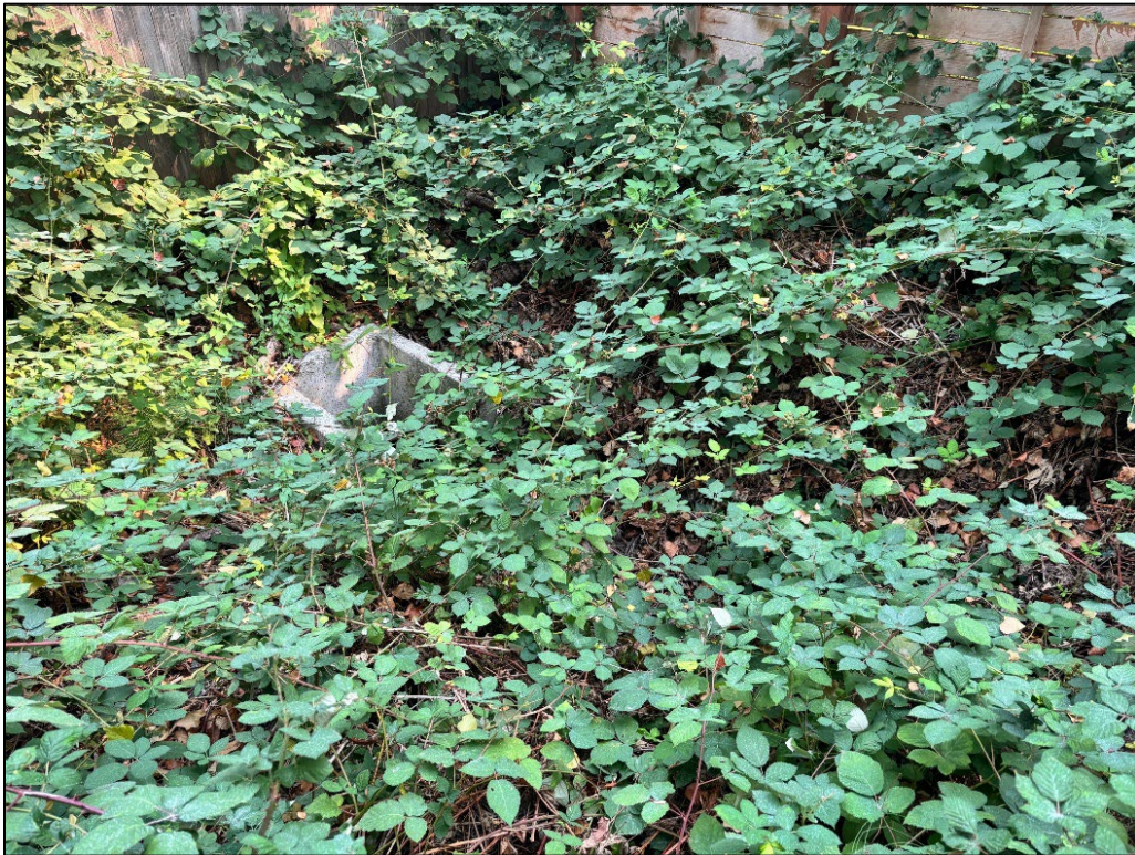
Figure 4. Vertical box culvert at end of open ditch in northeast corner of subject property
